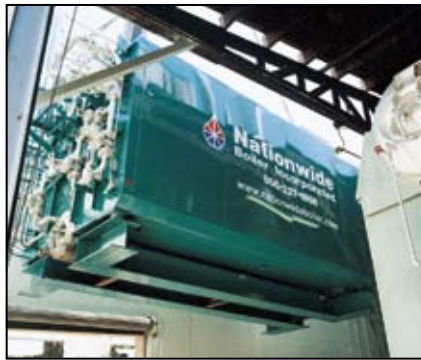
50,000 lb/hr package boiler with ultra low NOx burner being lowered into boiler room at Cribari Winery, Fresno, CA.
